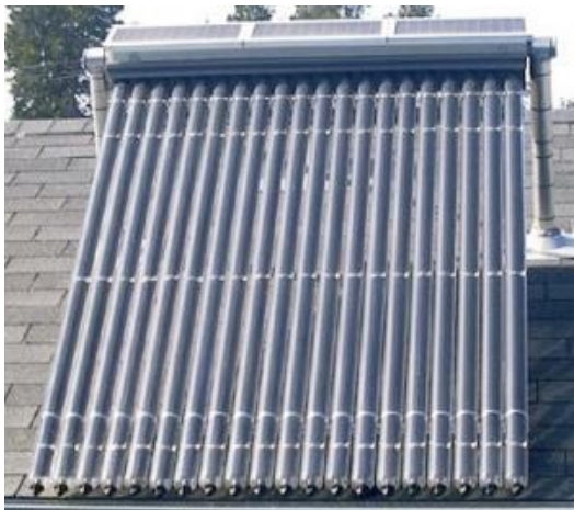
Solar hot water system
